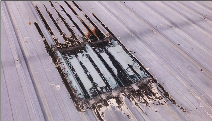
Another patched area.
