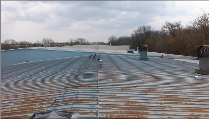
View looking East over rusted panels.
