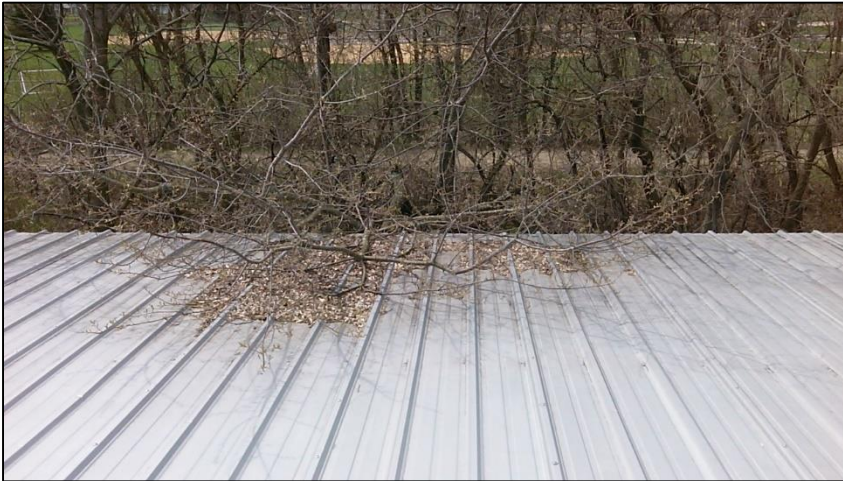
Tree laying on roof B South slope. This should be removed before more damage to roof panels occur.
