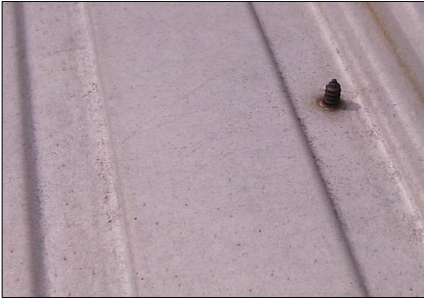
Screw from below coming up through roof panel.
